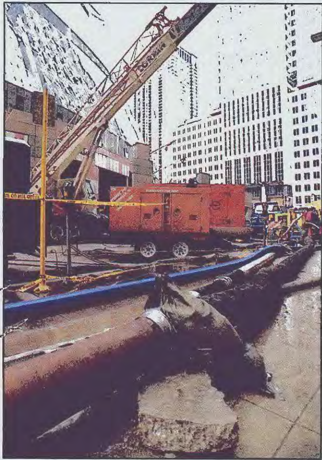
Water hoses and electrical equipment litter Chicago's Loop in an effort to pump out flooded basements.
