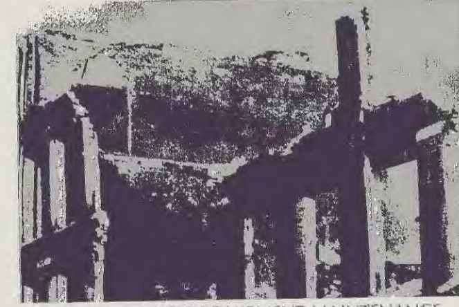
Cause: POOR EQUIPMENT MAINTENANCE
