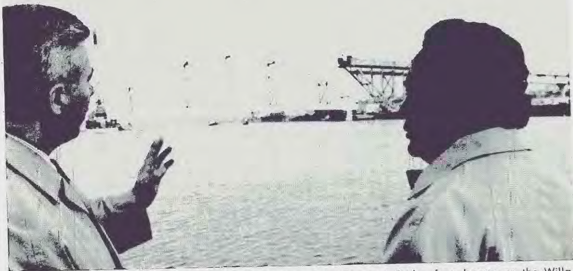
Hydraulic jacks begin lifting the 900-foot center section of the Fremont Bridge from barges on the Willamette River in Portland, Or. Watching are Phillip C. Monahan, INA, and Hans Davalos, of the agency.
