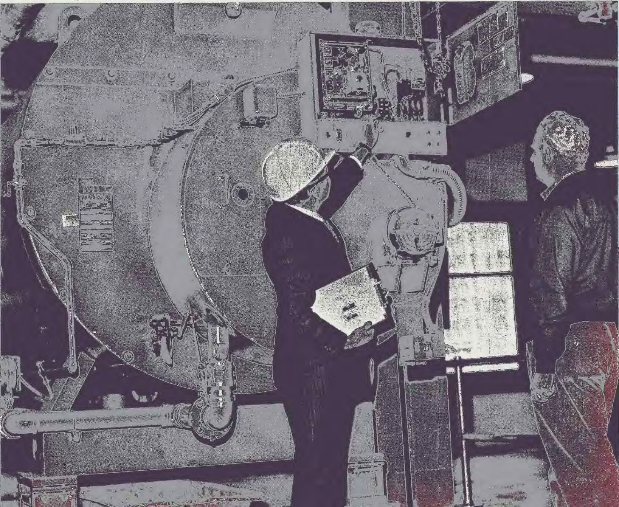
Inspector checks controls of steam boiler
