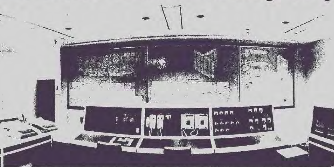
The elaborate fire safety system at the refurbished MGM Grand Hotel is monitored 24 hours a day.
