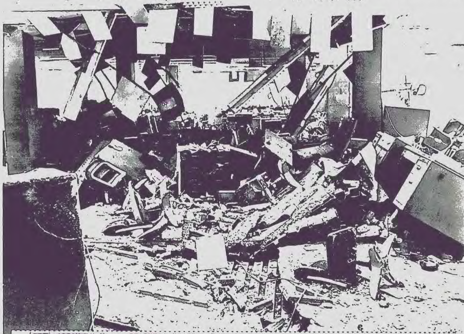
(REDACTED) N.Y., ---BUSINESS UPSET---This was the scene yesterday in the office of a local realtor after a boiler exploded in the room below. Floor and roof collapsed, destroying office equipment. There were no occupants in the building at the time of the accident. (REDACTED) (b1w638594/8571kp) 1967
