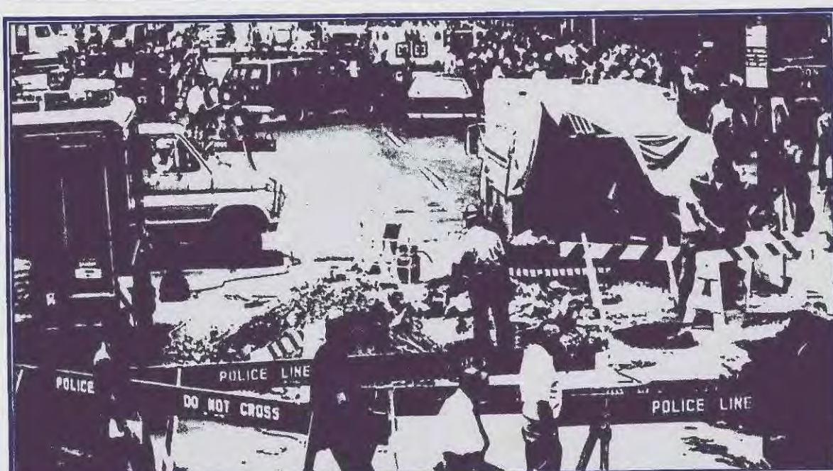
Photo: Wide World Consolidated Edison crews attempt to repair the underground damage that caused the chaos.
