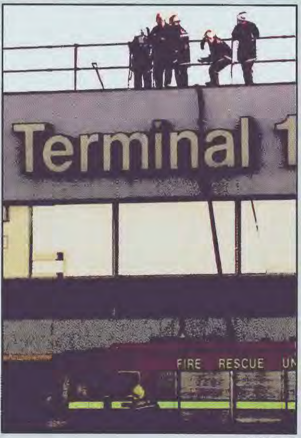
PHOTO: AFP The roof suffered most of the property damage from a recent fire at Heathrow Airport's Terminal 1.
