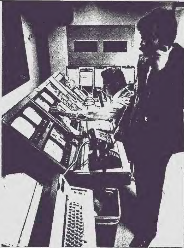
A sophisticated smoke detection system like this one at the Ritz-Carlton Hotel in Chicago could have averted the MGM tragedy.
