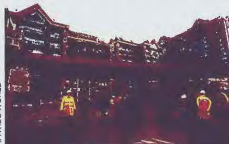
Falling glass prevented adjusters from getting to many buildings damaged in the Feb. 9 Docklands bombing.
