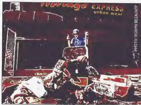
A worker clears debris from a clothing store in New Orleans damaged by Hurricane Katrina.
