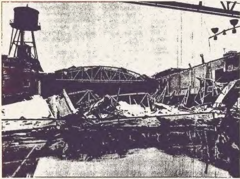
The tennis net stood firm while health club enthusiasts scrambled to safety when the roof of this Chicago club collapsed under a heavy burden of snow.
