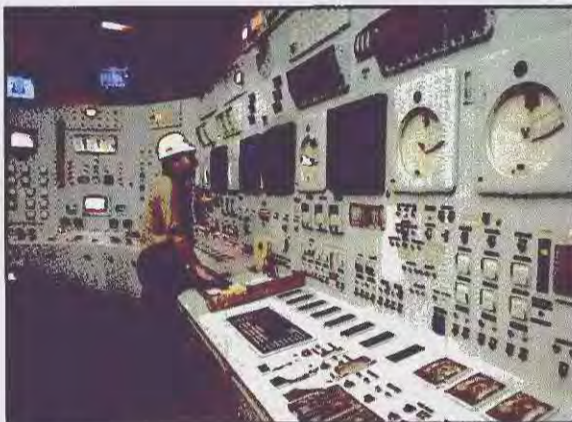
PHOTOS: AP/WIDE WORLD An engineer in the control room of the Moss Landing Power Plant in California, where the power grid remains close to crisis.
