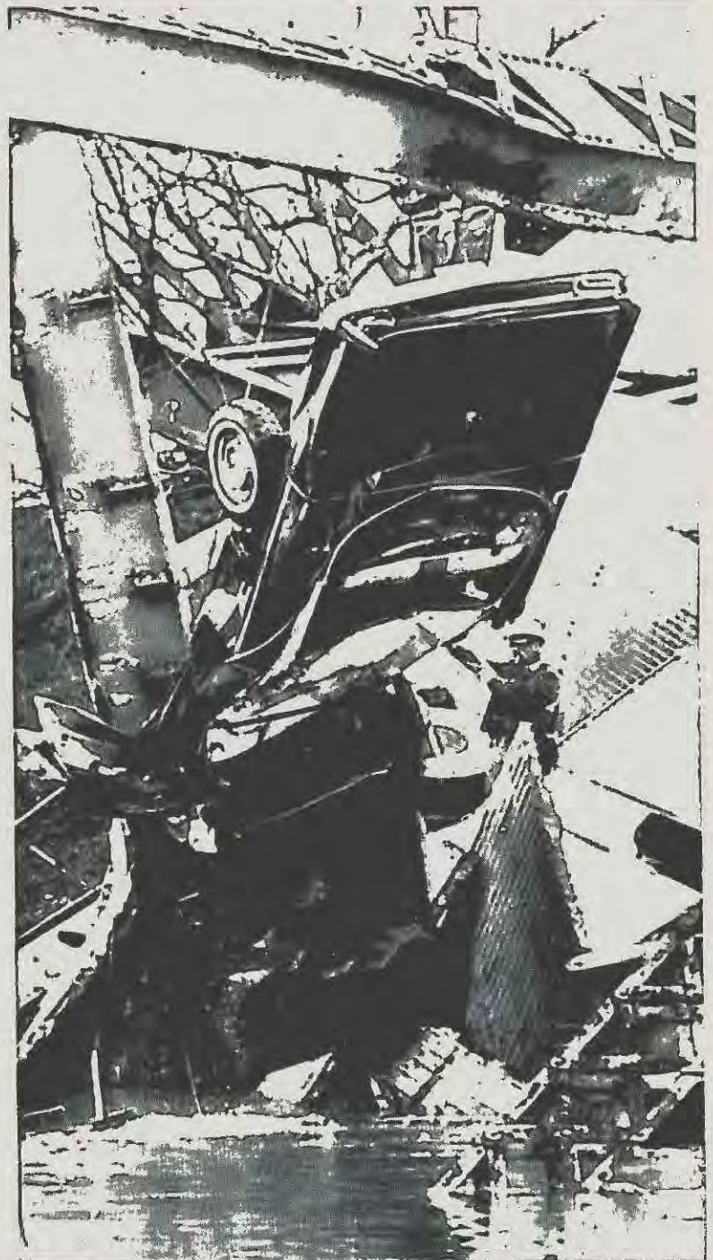
Tangled vehicles and structural steel tell the tragic story of the Point Pleasant Bridge collapse Dec. 15 that took at least 28 lives and destroyed scores of vehicles. The state of West Virginia, operator of the bridge, had no liability insurance coverage.
