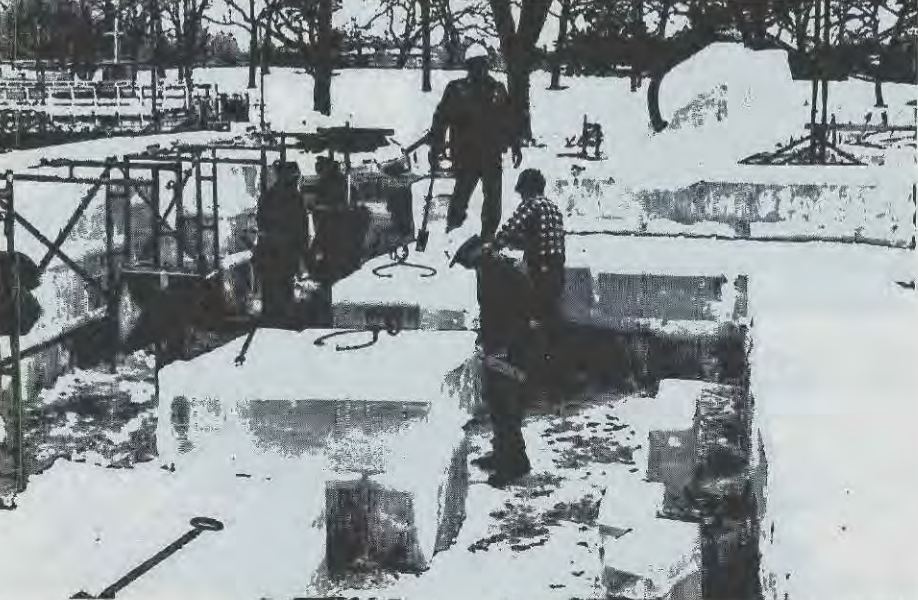
Work progresses on St. Paul's ice castle, which is the largest ever built. Photo: Silly Doroshov/St. Paul Pioneer Press Dispatch
