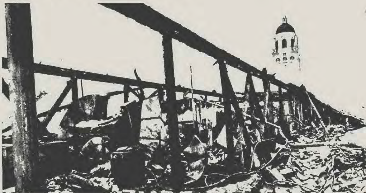
A protective sprinkler system was in the process of installation at the time of the fire that caused nearly $1 million damage to Stanford University's Encina Hall. —Wide World photo
