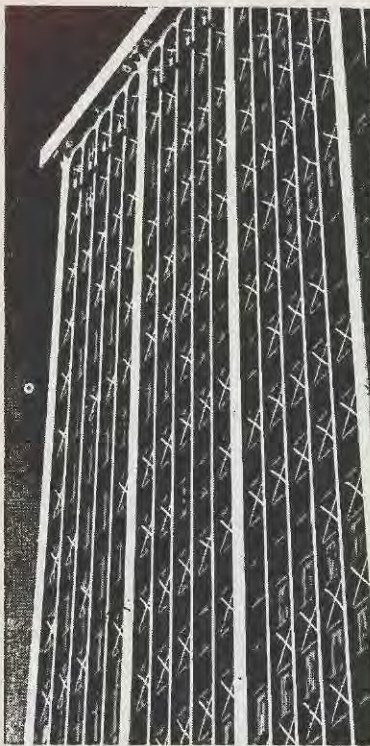
Windows have plunged from this bank facade to the sidewalk.
