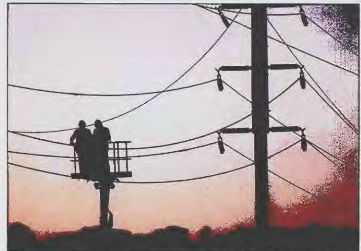
AP PHOTO Emergency cables have been installed to help supply power to central Auckland, New Zealand, where power has been out since Feb. 20.
