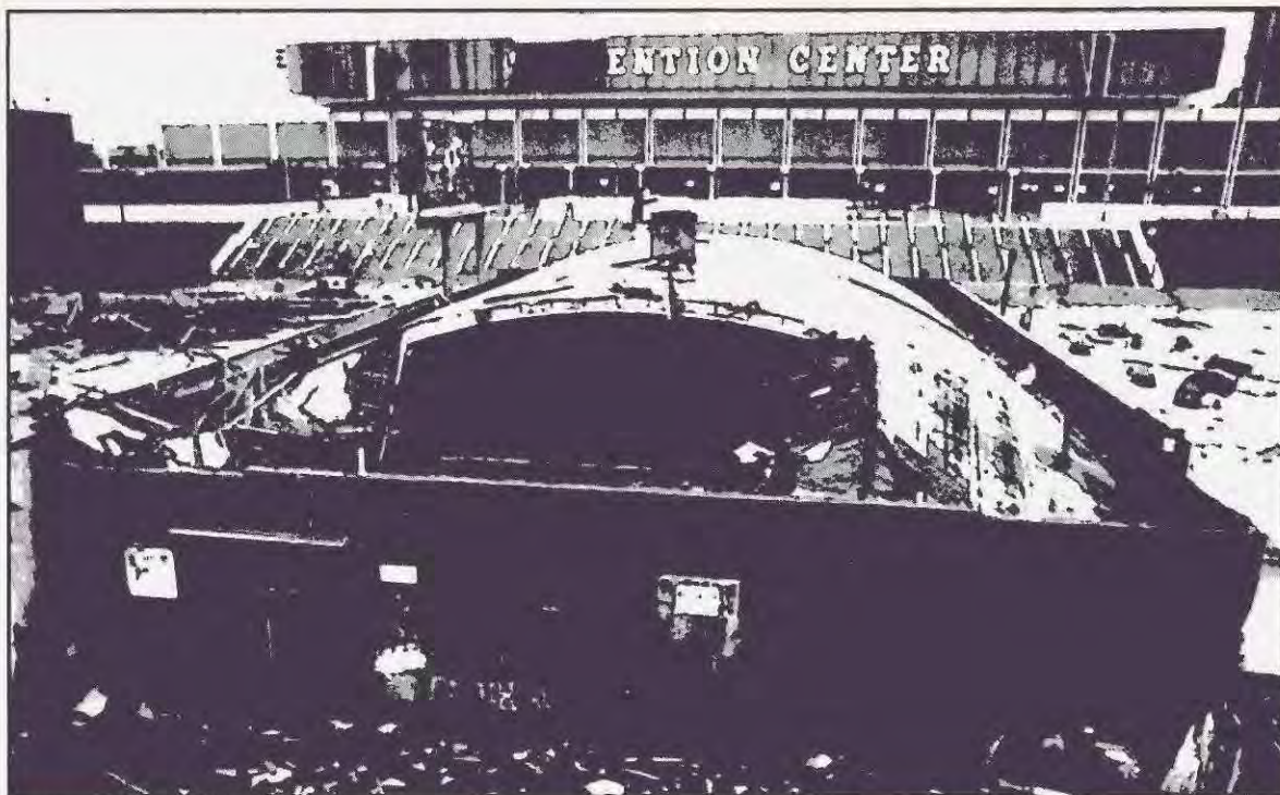
Photo: Wide World Last week's tornado tore a gaping hole in the roof of the Los Angeles Convention Center.
