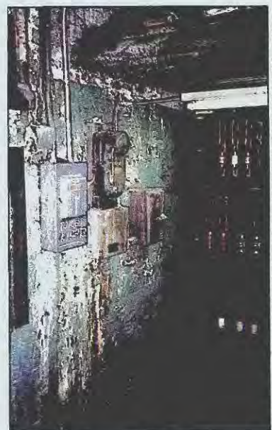
Hartford Steam Boiler will inspect the approximately 12,000 buildings it insures after finding potential electrical problems in a study.
