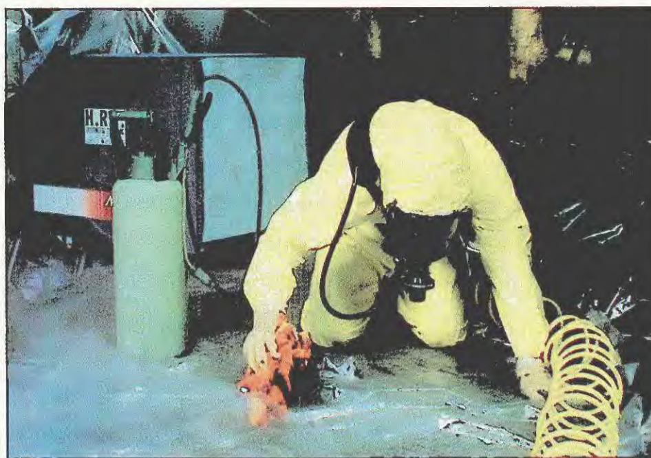
The need for asbestos abatement liability insurance is growing at exponential rates as the demand for asbestos removal increases. Photo: LVI Environmental Services Group Inc.
