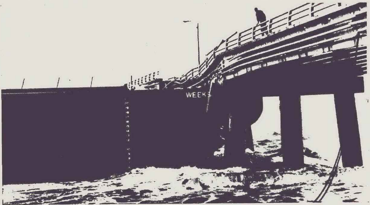
An empty 235-foot barge rammed into the Chesapeake Bay Bridge-Tunnel late last month, causing an estimated $1,150,000 in damage. —World Wide photo
