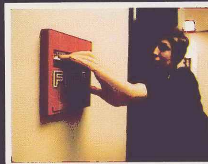
Manual stations, located near exits, permit occupants to turn in alarm. Often include a 2-way intercom for on-the-spot reporting.
