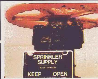
All sprinkler shut-off valves are supervised to warn when water supply has been cut off.
