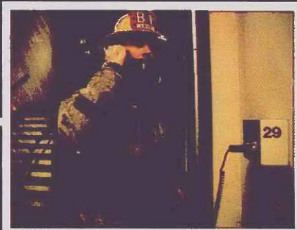
2-way intercom serves as vital communications link between commander and firefighters.
