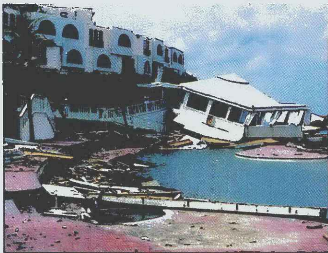
On St. Croix, one of the storm-wracked islands, a formerly poolside restaurant bore the brunt of Hurricane Marilyn.
