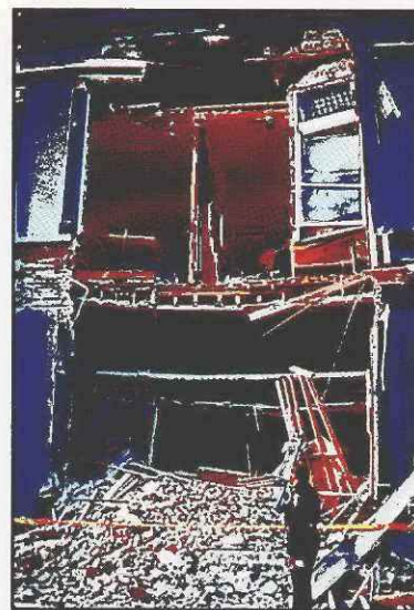
PHOTO: H.G. WILSHIRE/U.S. GEOLOGICAL SURVEY Masonry structures such as this one suffered some of the worst damage in the 1989 San Francisco quake.
