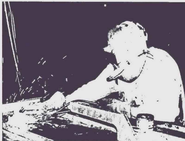
Worker welds a piece of steel. OSHA is watching through the use of a portable air-sampling instrument running through tube at the mouth.
