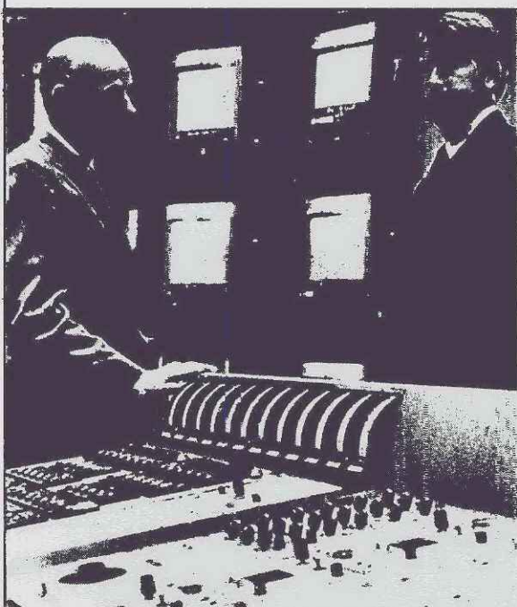
Photo: Steve Sherwood Olice Steward, left, and Dennis Wales talk in the utility's master control room.
