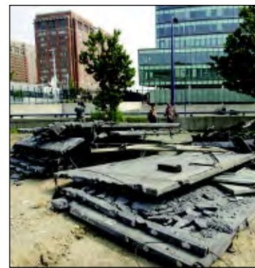
A $458 million settlement was reached in the collapse of a highway tunnel on I-90 in Boston.
