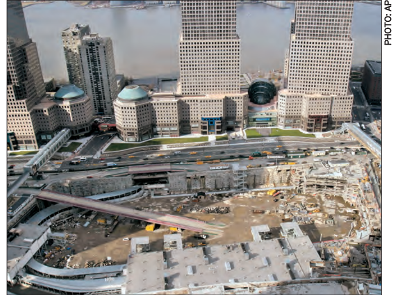
The 16-acre site where the World Trade Center stood is scheduled for redevelopment.
