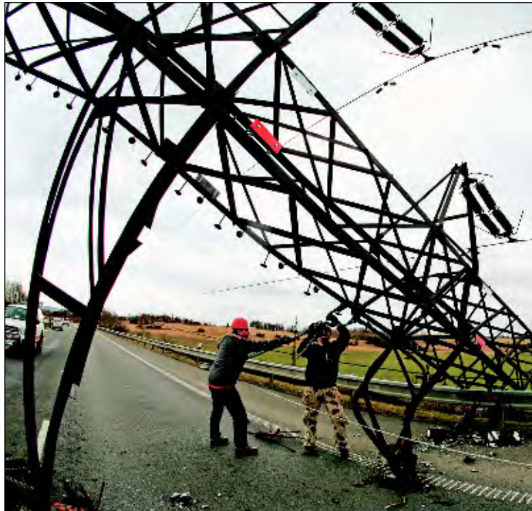
Workers remove wires from a high-voltage tower that toppled across a roadway in Mlada Boleslav, Czech Republic, northeast of Prague when Windstorm Emma produced high winds and heavy rain March 1 across much of Europe.
