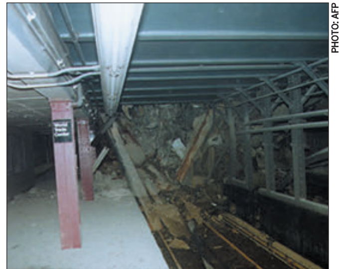
Debris from the collapse of the World Trade Center's twin towers crashed through the ceiling of New York City Transit's Cortlandt Street subway station, located beneath the center.
