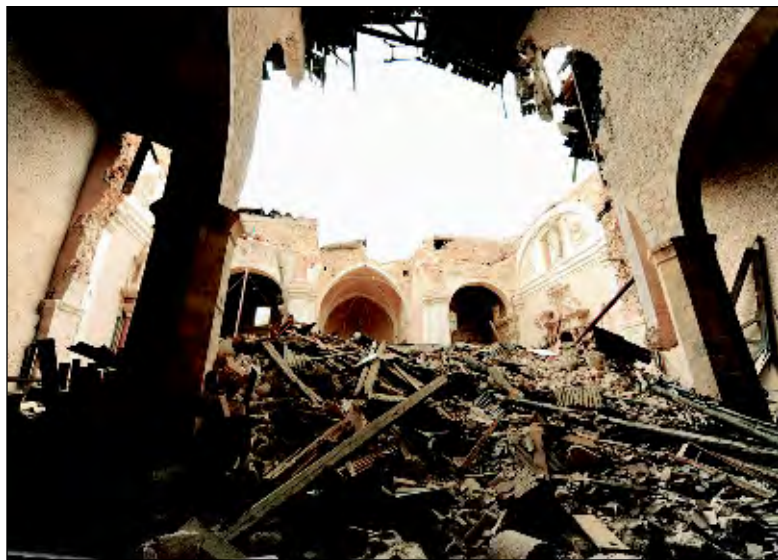
Rubble remains inside Santa Maria of Collemaggio Basilica in L'Aquila, Italy, a 15th century structure, a week after a major earthquake struck the region.
