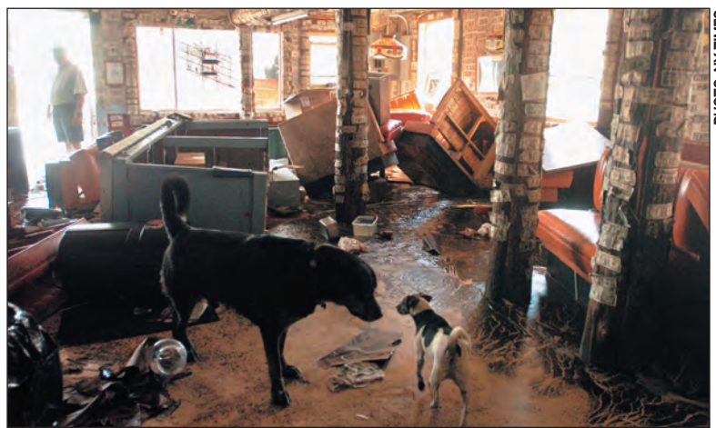
Hurricane Dennis, which packed 120 mph sustained winds, hit the Florida Panhandle, causing damage to some properties.
