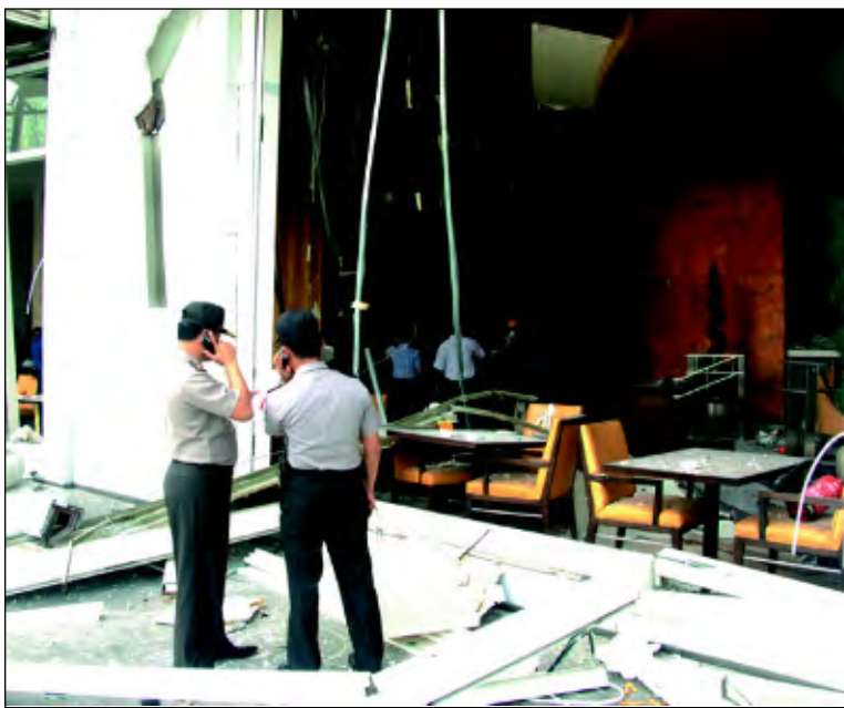
Police officers inspect damage at the Ritz-Carlton hotel after bombs exploded in Jakarta, Indonesia, on Friday.
