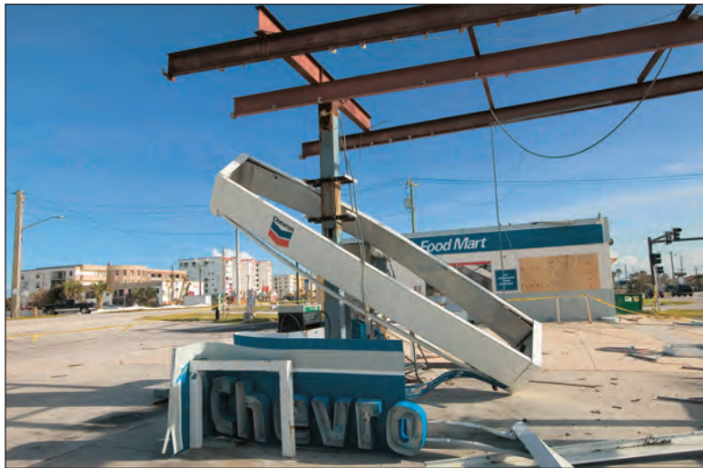
Widespread damage from Hurricane Frances and the other three storms that hit Florida last year created a surge in demand for good and services related to repairs.
