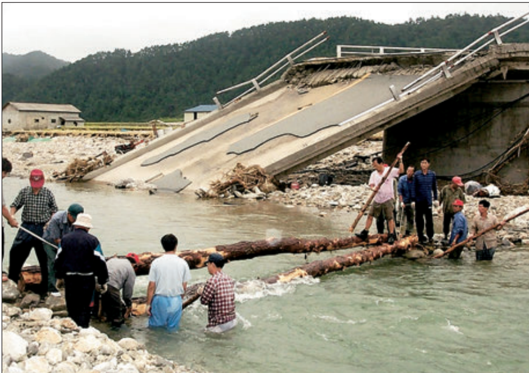
Workers build a log foot bridge across a South Korean river after Typhoon Rusa, which caused an estimated $835.5 million in property damage, knocked out a bridge.
