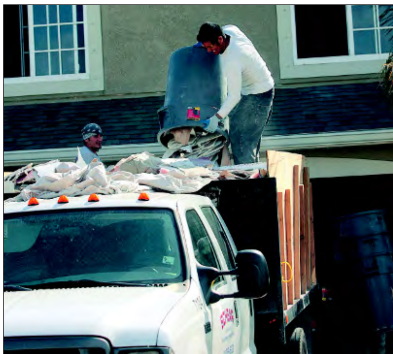
Workers remove contaminated drywall from a home in Bradenton, Fla., in January 2009. Litigation against a China-based drywall maker continues.
