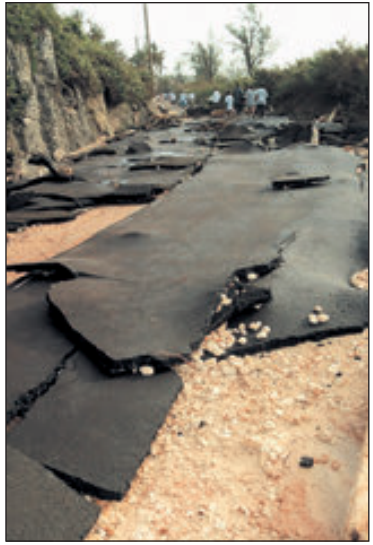
Bermuda continues to repair damage, such as this buckled road, from Hurricane Fabian.
