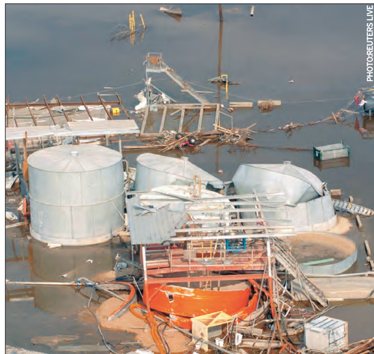
Oil storage tanks in Cameron, La., were heavily damaged by Hurricane Rita.
