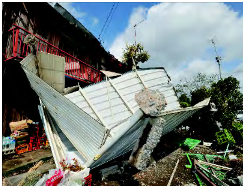
Buildings in central Japan were battered by Typhoon Melor last week. Insured losses were blunted by good quality construction of many buildings in the region, according to catastrophe modeler AIR Worldwide.
