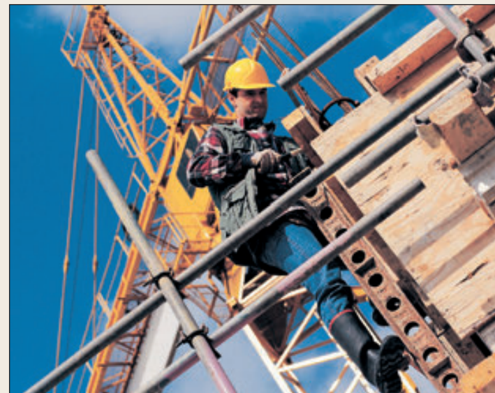
New York's scaffold laws, designed to protect workers, are contributing to climbing liability rates in the state.
