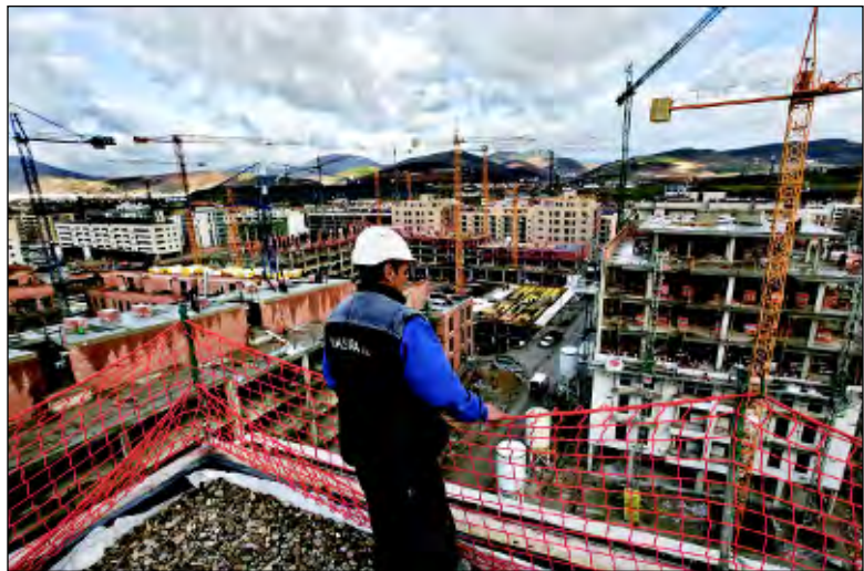
AP PHOTOS A worker eyes a construction project last December in Pamplona, Spain, where a drop in building has major construction companies concerned about reasonably priced coverage and underwriters worried about shareholder litigation.
